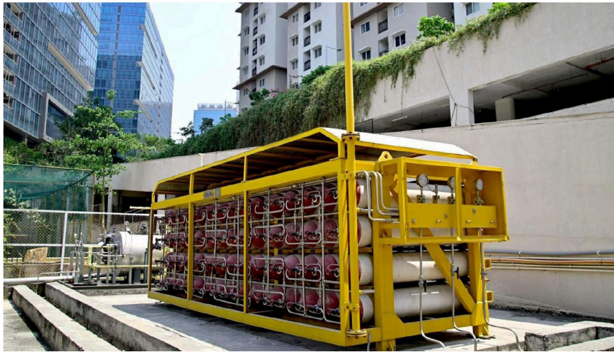
A decompressor unit installed at Prestige High Fields, as part of the piped natural gas (PNG) infrastructure that regulates gas pressure for safe distribution at the gated community in Hyderabad, a resident operating a PNG meter at Malaysian Township in Hyderabad. scowari / ianxun
