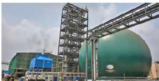
Energy security: The compressed biogas plant at Brahmapuram currently processes about 50 tonne of biodegradable waste a day.
