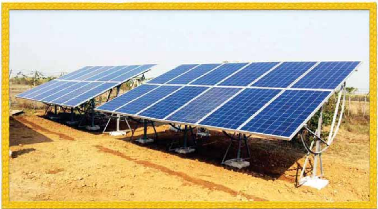
Natural Gas based Closed circuit Vapour Turbine replaced by Solar Power at Dibiypur Compressor Station in Uttar Pradesh
