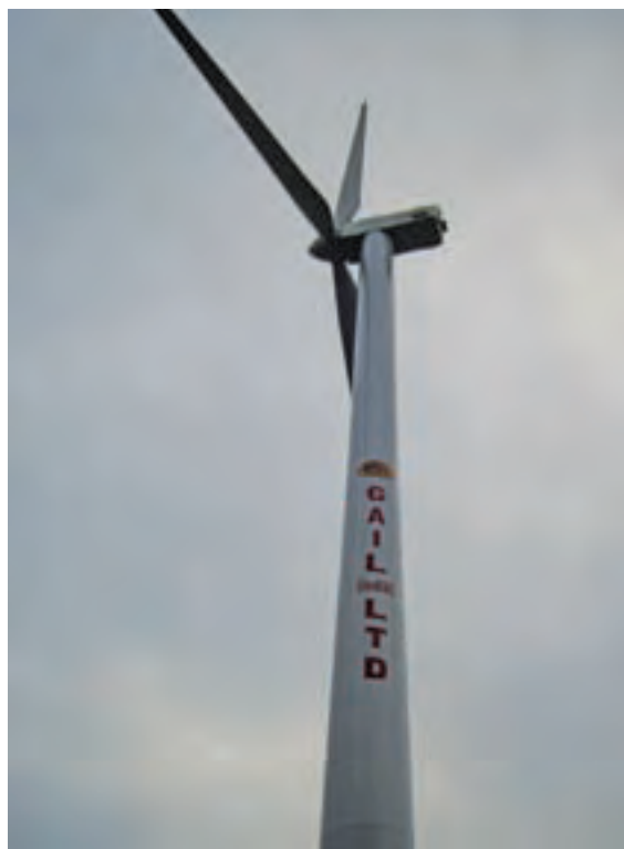
GAIL's Wind Power Installation
