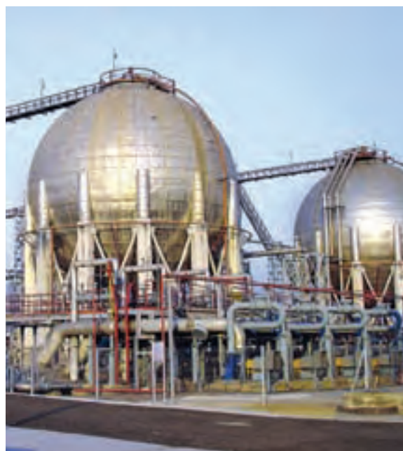
Horton Sphere LPG Storage Tank at GAIL Installation
