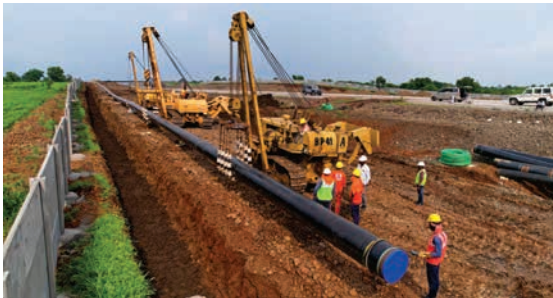
Laying of Natural Gas pipeline from Mumbai to Nagpur under MNJPL project
