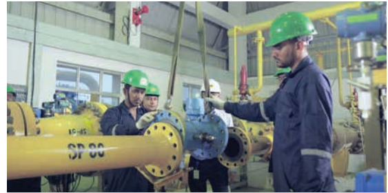
Meter Prover Facility at GAIL, Hazira
