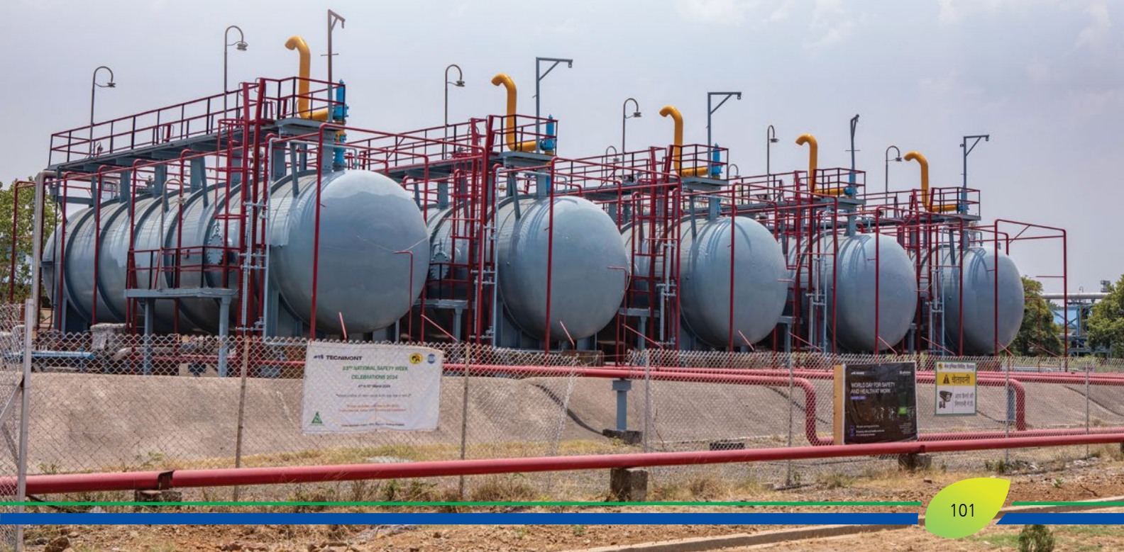
10 MW Green Hydrogen Plant in GAIL, Vijaipur
