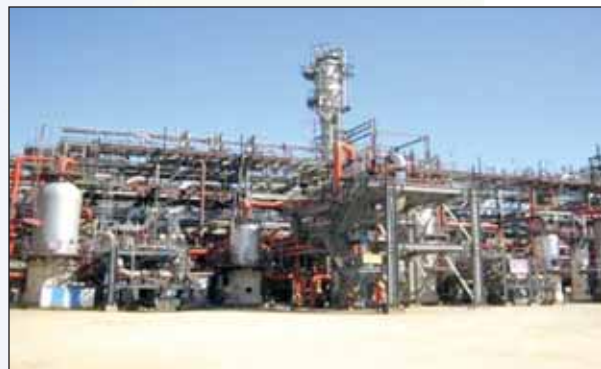
Gas Sweetening & C2+ Recovery Unit
