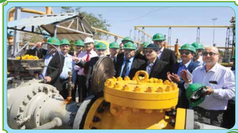
Diversion of GNAQ gas to GPU Gandhar through 24" HP pipeline GNAQ gas charging in New HP Line carried out.
