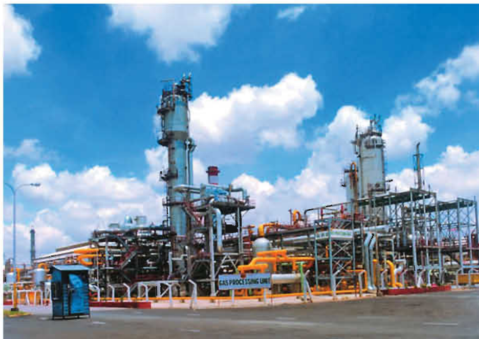
Gas Processing Unit at GAIL, Pata, U.P.
