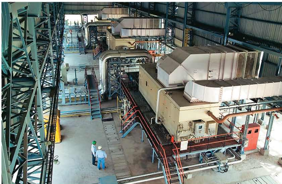
Gas Turbine at GAIL, Vijalpur, M.P.
