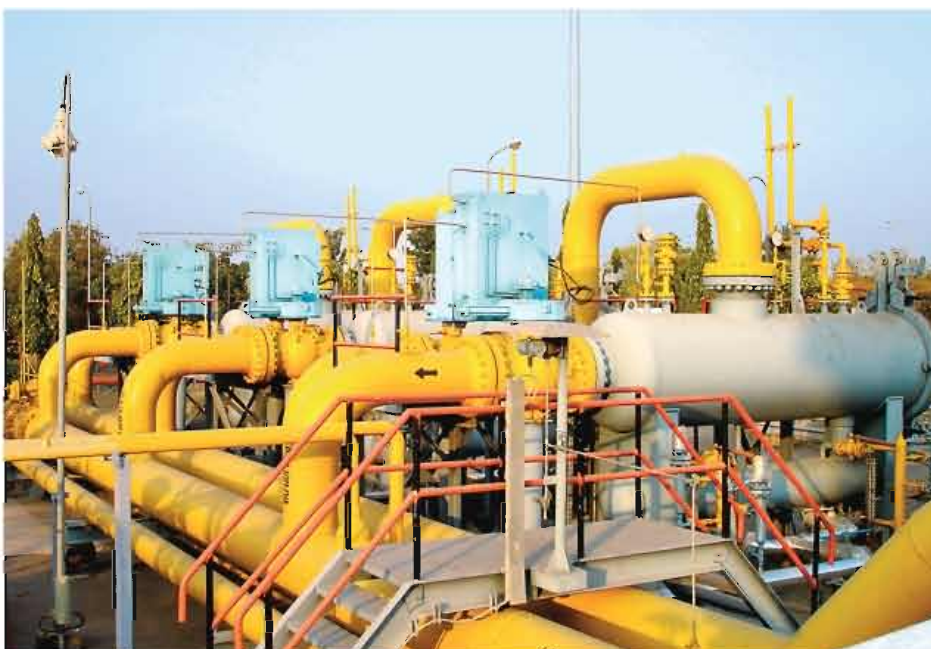
Gas Terminal, Dibiyapur, Auraiya, U.P.
