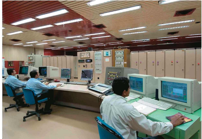
Control Room in a LPG plant
